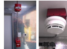
◀ Full fire alarm system with pull stations and smoke detectors
